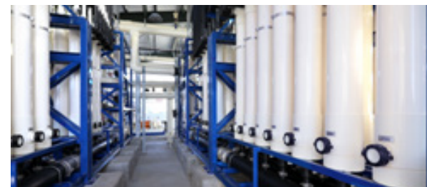
December marked one year on from the official opening of The Claude "Bud" Lewis Desalination Plant in Carlsbad. The city just completed a project to nearly double the size of the facility.
